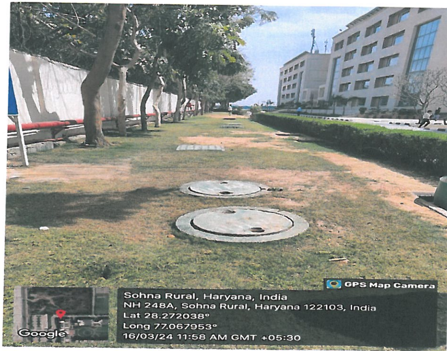
Image: Rainwater harvesting pits
