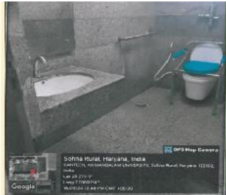
Accessible toilet facility for differently-abled individuals
