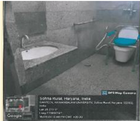
Accessible toilet facility for differently-abled individuals
