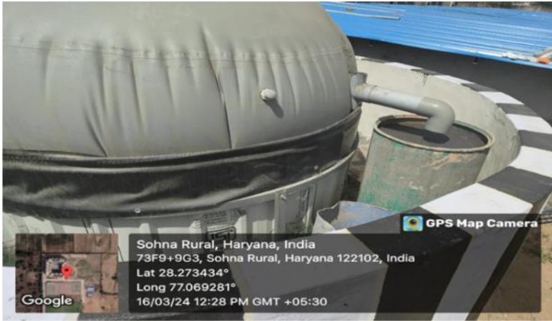
Biogas outlet & slurry discharge used as organic manure for campus horticulture sustainability
